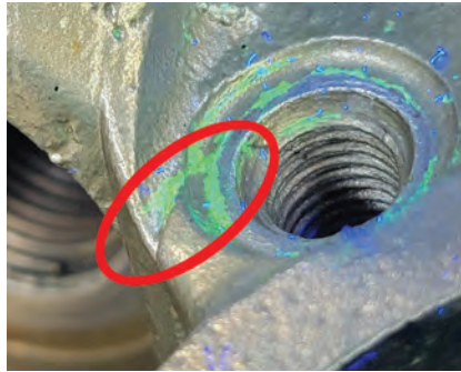
Fluorescent dye penetrant inspection. This might or might not be a crack. If it is a crack, it doesn't present a safety issue.
